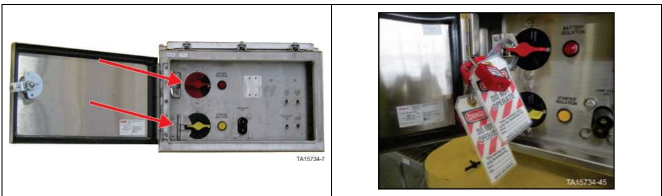
Figure 31. Battery Isolation Box – Battery isolation switch in OFF position with locks in place
