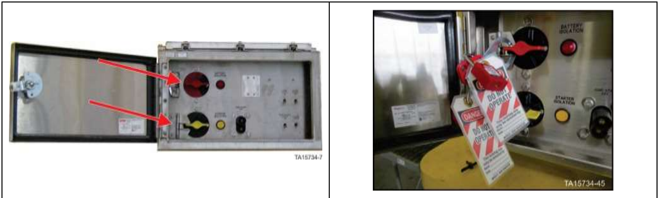
Figure 33. Battery Isolation Box – Battery isolation switch in OFF position with locks in place
