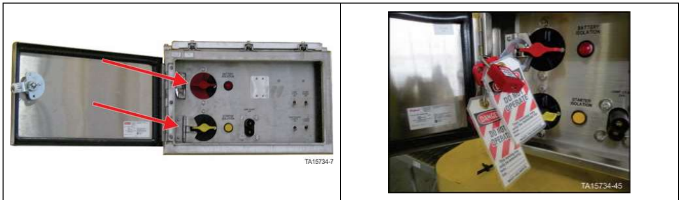
Figure 5. Battery Isolation Box – Battery isolation switch in OFF position with locks in place
